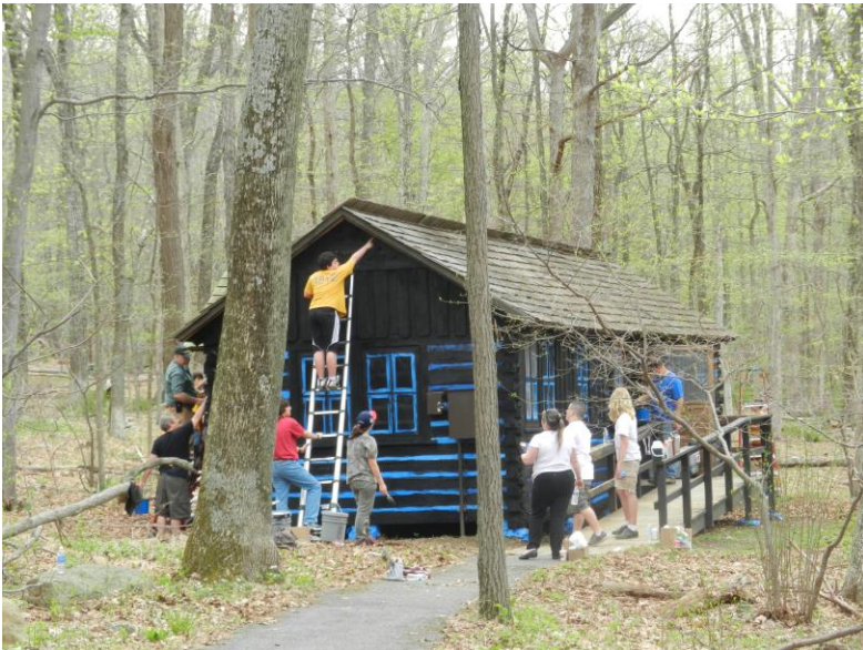
The chinking between the logs received blue painter's tape and then the logs were stained.
